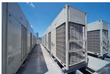
VRV Q installation
