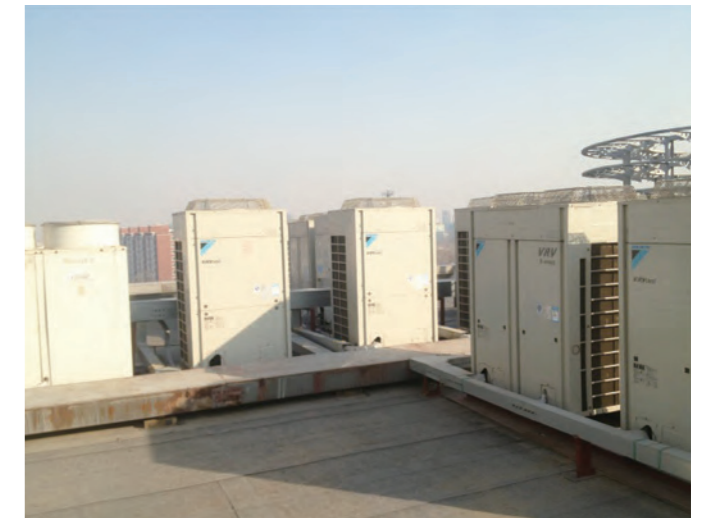
After VRV Q installation
