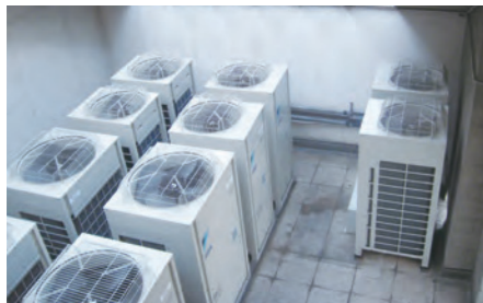
The original VRV units that ran on R22 were replaced with VRV III-Q units running on R410A.
