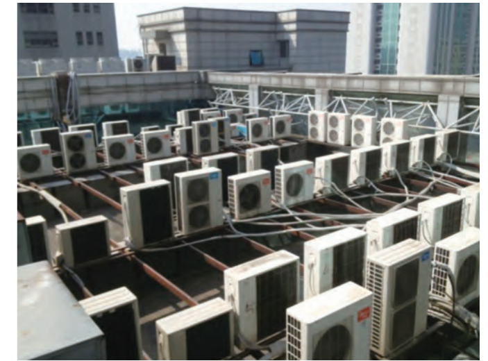
Before Multiple brands installed
